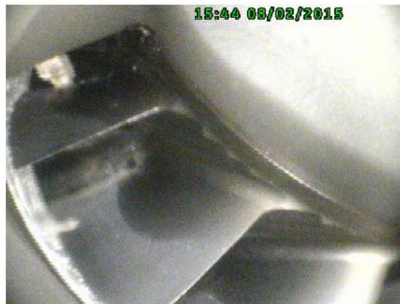
Photo No. 14 High pressure impeller.
