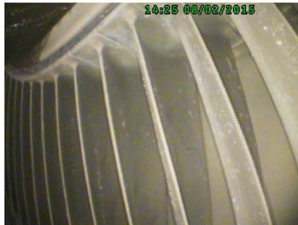
Photo No. 39 First stage power turbine.
