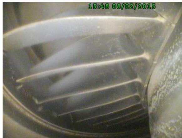
Photo No. 9 Low pressure turbine.
