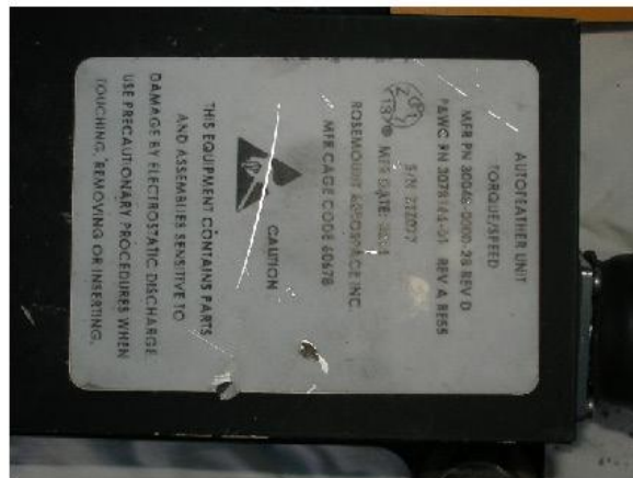
Photo No. 23 Autofeather unit data plate.
