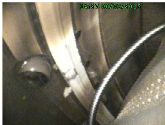
Photo No. 44 Combustion chamber liner.
