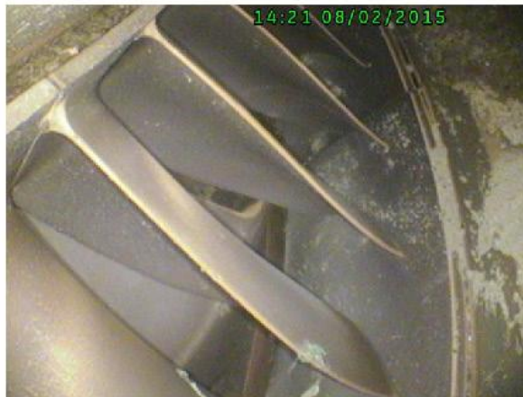
Photo No. 41 Low pressure turbine.
