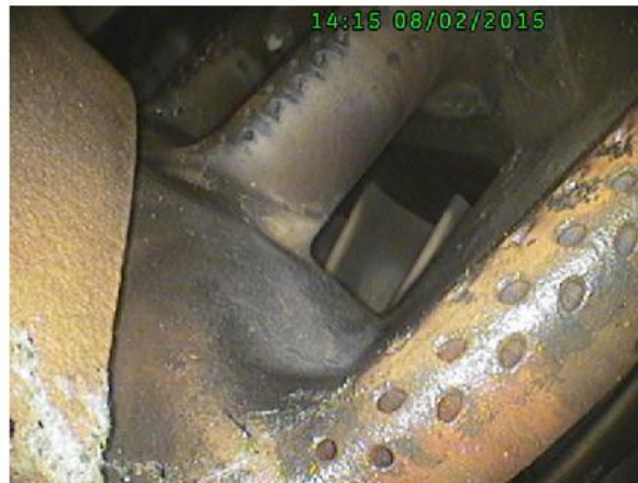
Photo No. 43 High pressure turbine vane ring.
