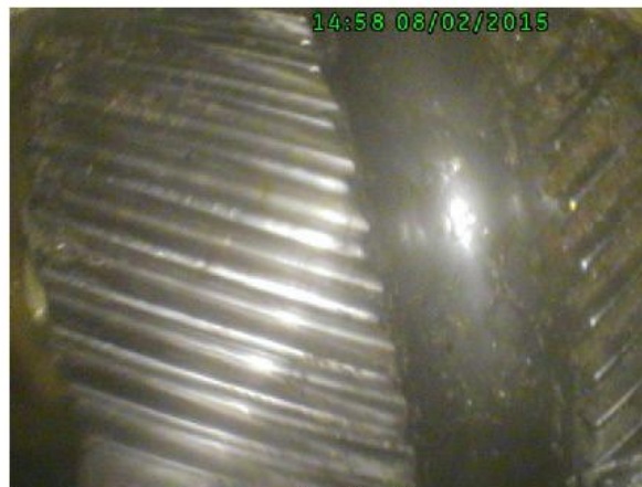
Photo No. 48 Reduction gearbox helical gear, detail.
