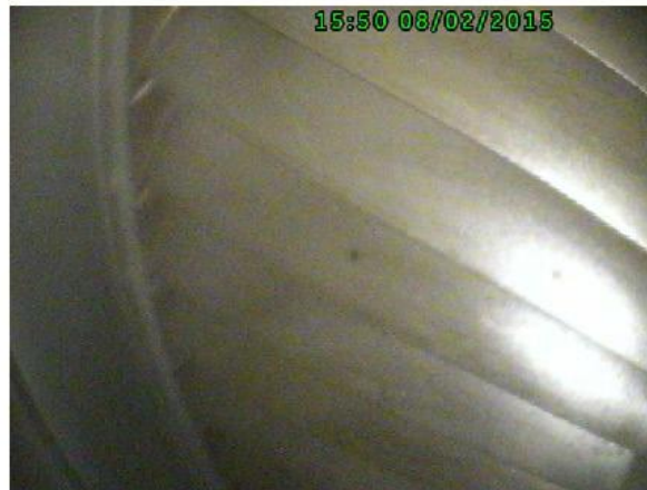
Photo No. 6 Second stage power turbine.
