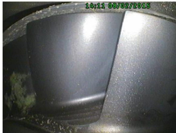
Photo No. 46 High pressure impeller.
