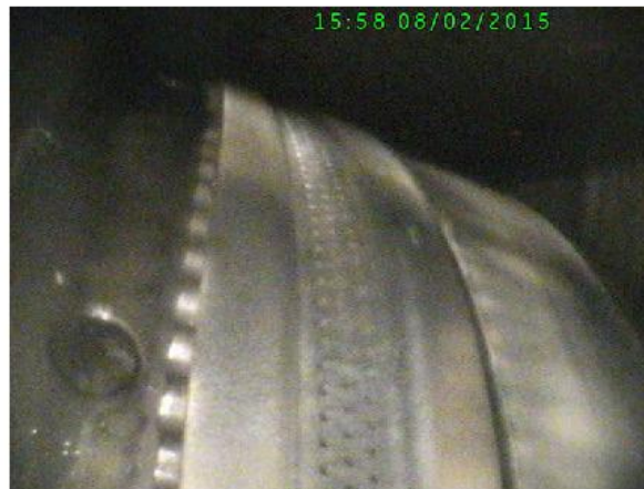
Photo No. 12 Combustion chamber liner.
